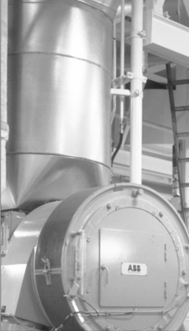
FUEL & LUBE OIL CABINET
