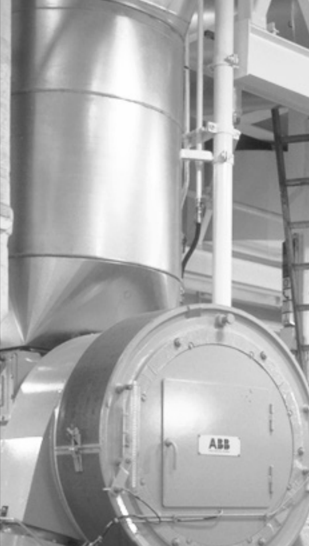
FUEL & LUBE OIL CABINET
