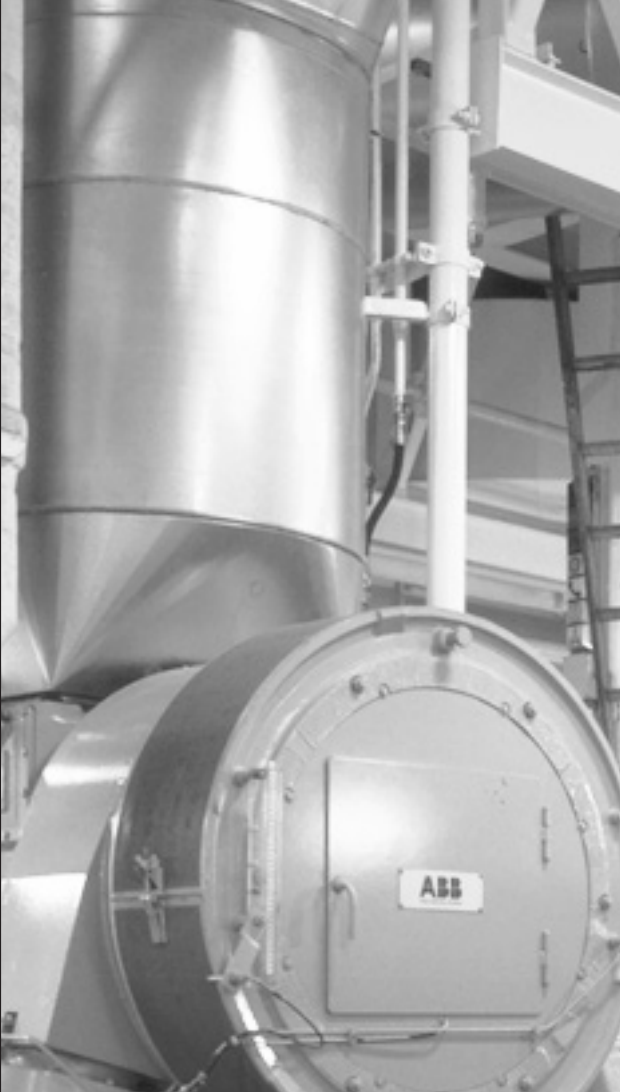
FUEL & LUBE OIL CABINET
